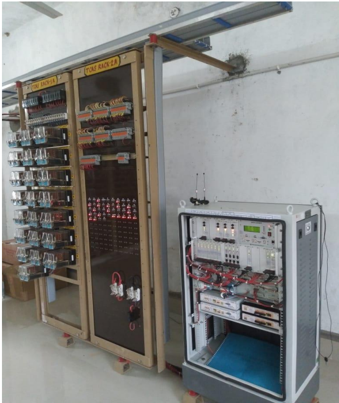
Station Kavach and Relay Racks
